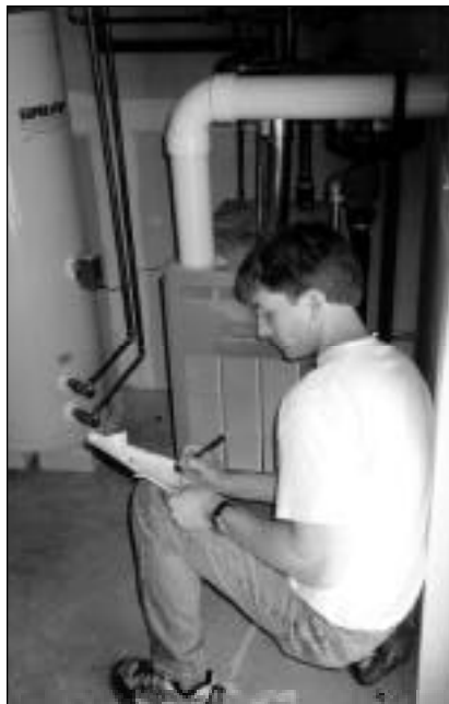
Home energy rater Pat Haller, of the Vermont Investment Corporation, checks the efficiency of this furnace and water heater.
