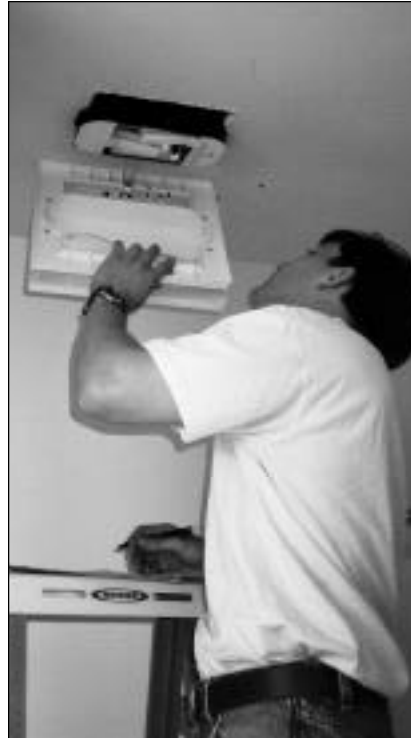
The types of light fixture found in a house have an effect on annual energy use. Here, Haller checks a bathroom fixture.
